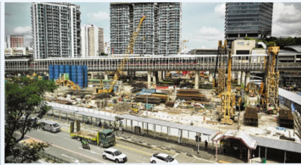
The site of the future Jurong East Integrated Transport Hub, which will house Jurong Regional Library as well as a community club, a sports centre, offices and retail space. ST PHOTO: LIM YAUHUI
