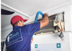
A technician with Wia Aircore Services, which has seen urgent requests for servicing increase by 40 per cent in the past three months, working on an overhaul of the air-conditioning system. It also has to undertake more extensive work such as cleaning air-con pipes and condensers almost daily.
